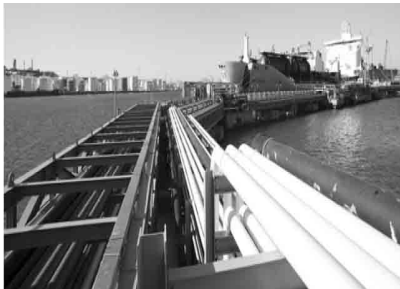
Ship to Ship T/S (Double Banking, Cross Jetty)
